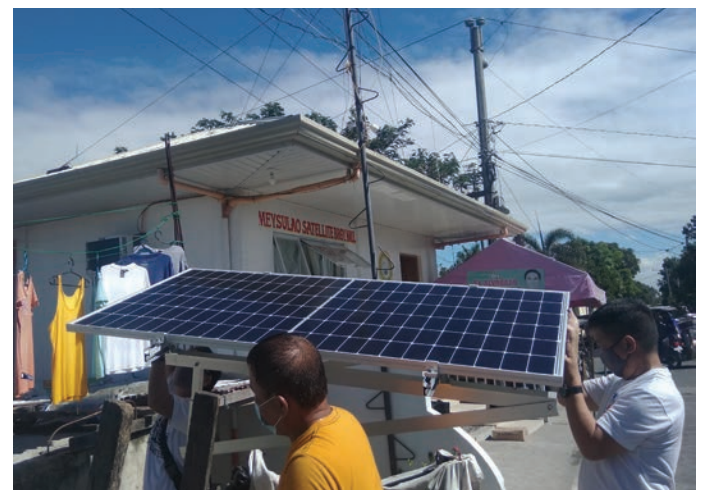
▲ CREST installed an emergency solar PV system to power Meysulao DRR Center.
