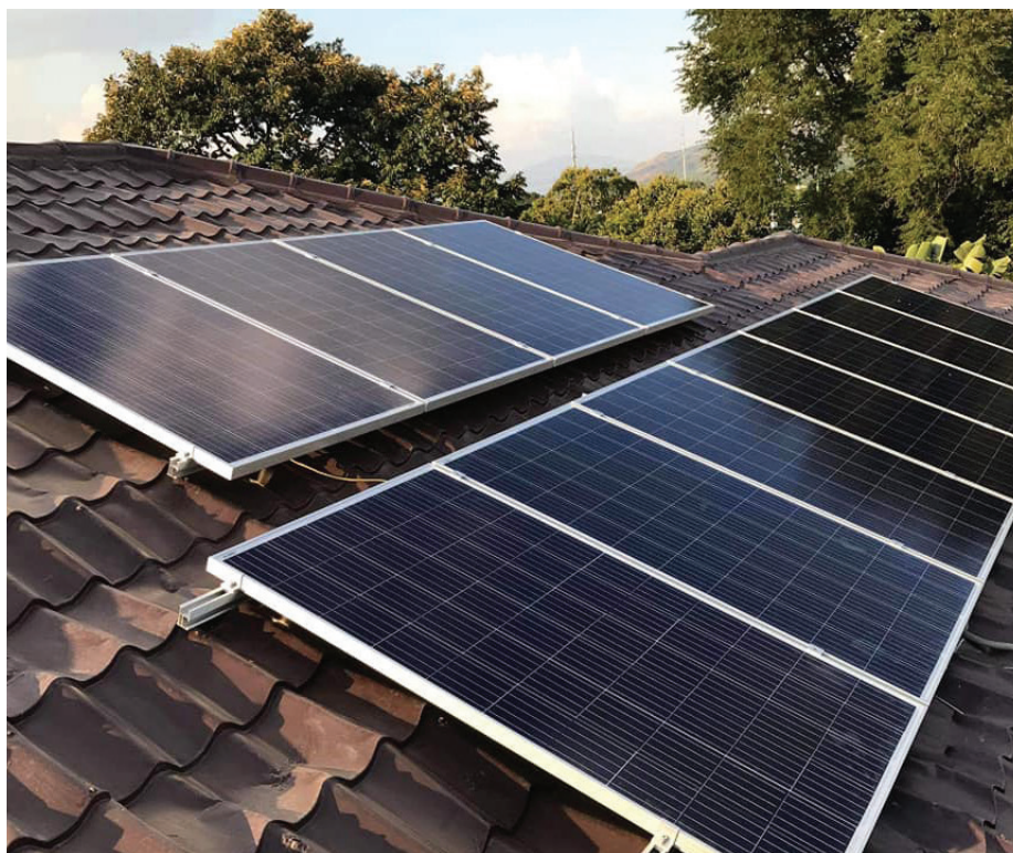
▲ Solar PV rooftop
